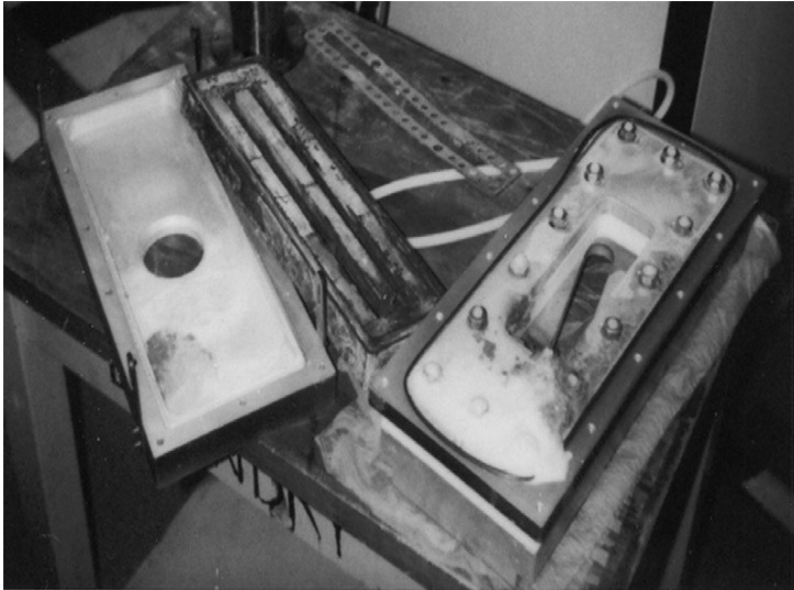
Figure 20.20 A photograph showing the corrosion products, the white foam-like material, that has overgrown the “O” ring.
